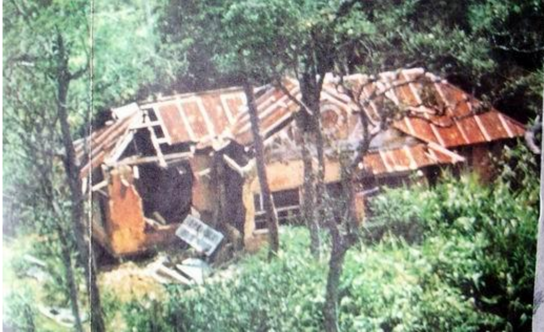
Figure 5- 1 A steel roof on a damaged house in 1969 (photo in Higl 1969)
